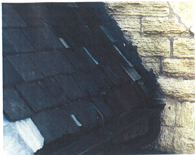
Areas of the slate roof had little or no flashing, and had been repaired a number of times in the past. Many of the slate roofing pieces had been turned over and re-laid, and a few were broken or missing.
