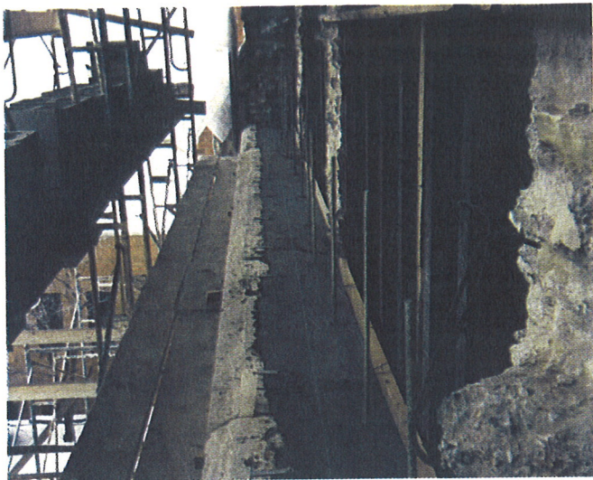
Before the stone at the west wall was re-installed, workers poured a reinforced concrete beam the full length of the west wall, from which block backup wall was built.
