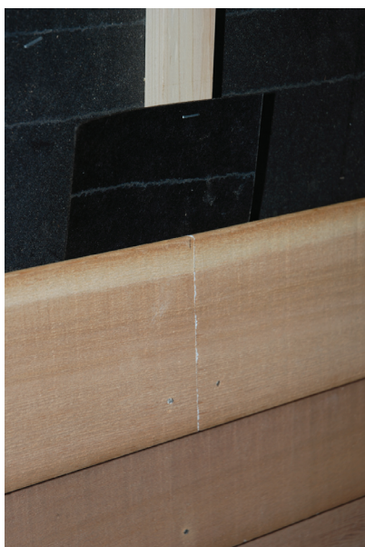
Figure 6—Completed joint. Note that fasteners are approximately one inch (25 mm) from the bottom edge of the siding and spaced well away from the end of each board. Nails were angled slightly to penetrate the furring strip and the underlying sheathing and wall stud.
