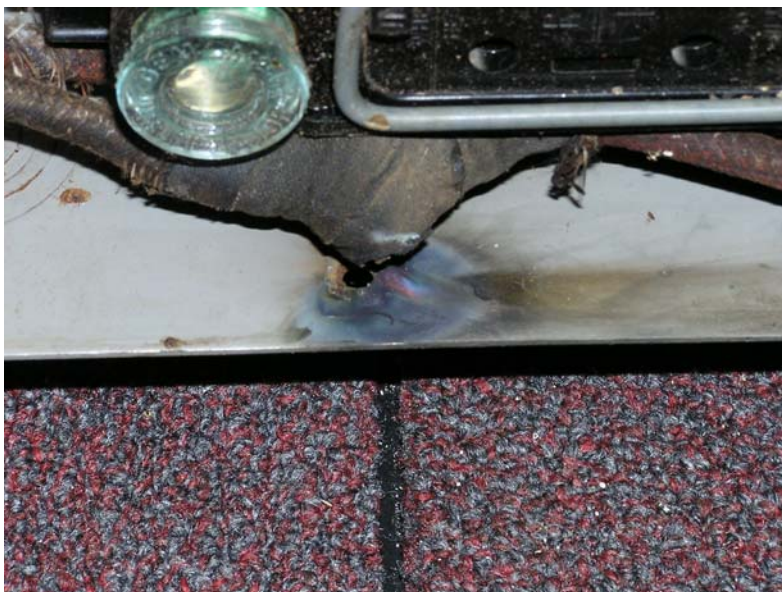
Fig. 9 – Arcing at Conductor Splice at House WI-1
