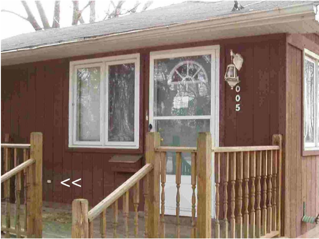
Fig. 25a– House IL-5, Non-Operational GFCI Receptacle With No Outdoor Faceplate or Box Cover
