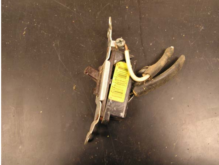
Fig. 32 – House TX-1, White Colored Grounding Conductor
