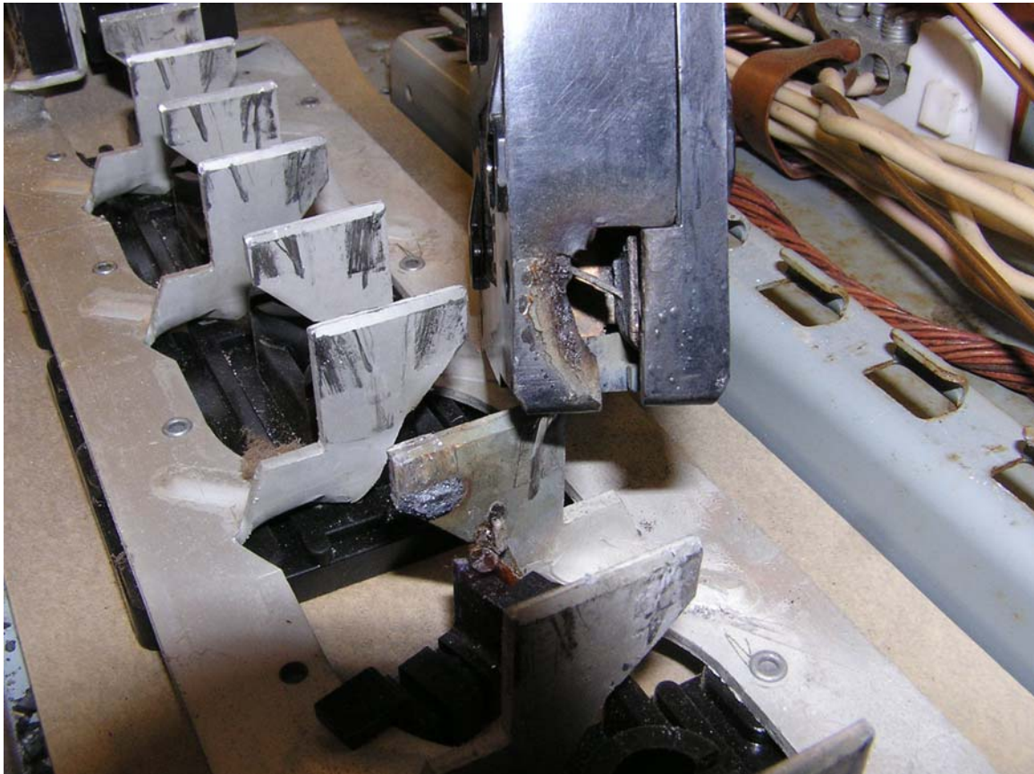
Fig. 11 – Arcing Damage at Breaker Stab at House MA-3
