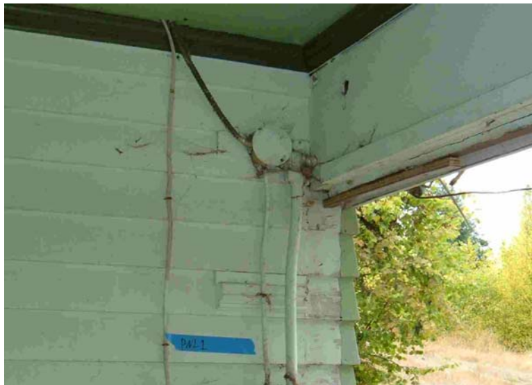
Fig. 37 – House OR-1, AC Cable Installed Outdoors
