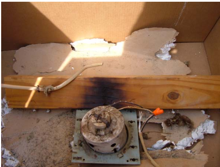
Fig. 43b – House AL-6, Recovered Recessed Ceiling Luminaire
