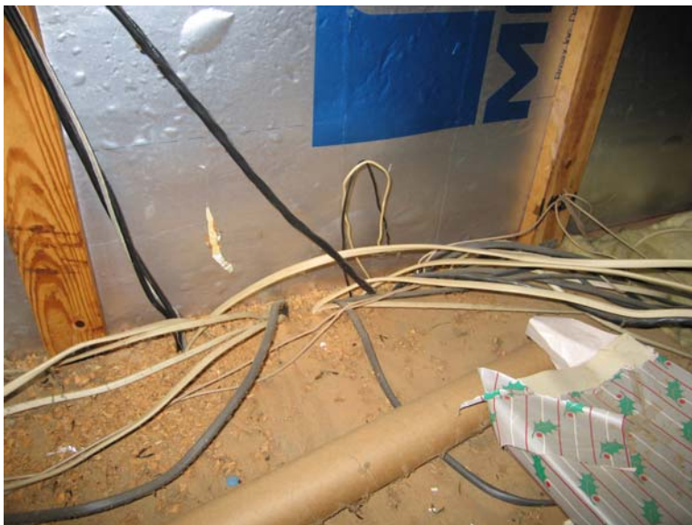
Fig. 39 – House VA-1, NM Cable Not Supported by Staples
