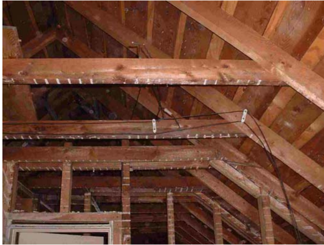
Fig. 1b – Knob-and-Tube Wiring From House IL-6
