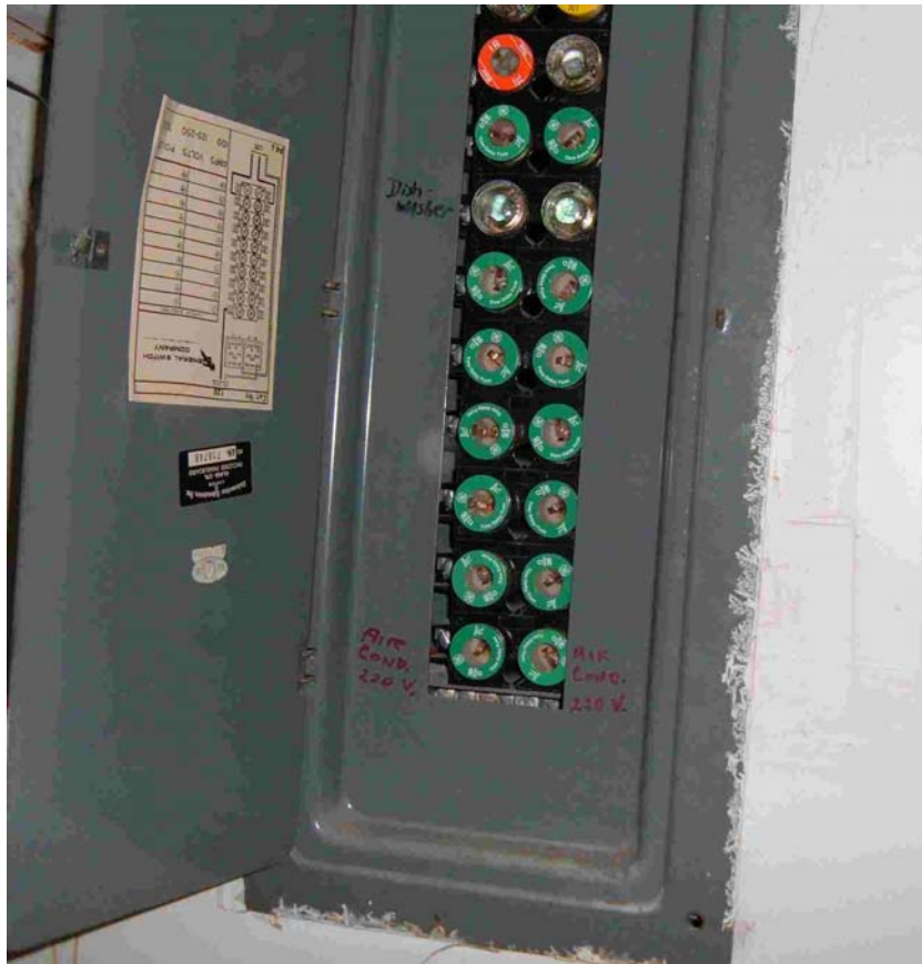
Fig. 12 – 30 Amp Fuses From House AL-8
