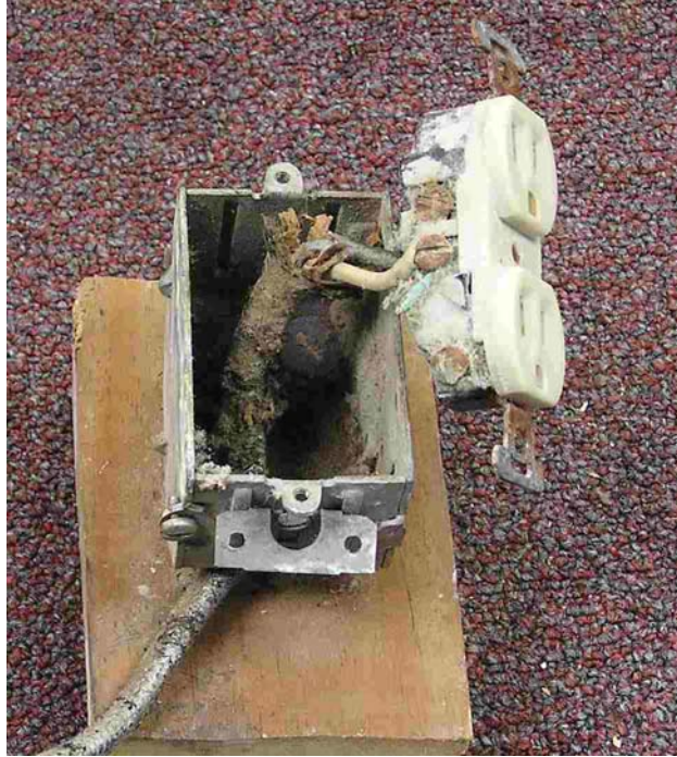
Fig. 41 – House AL-4, Grounding Type Receptacle Without Ground
