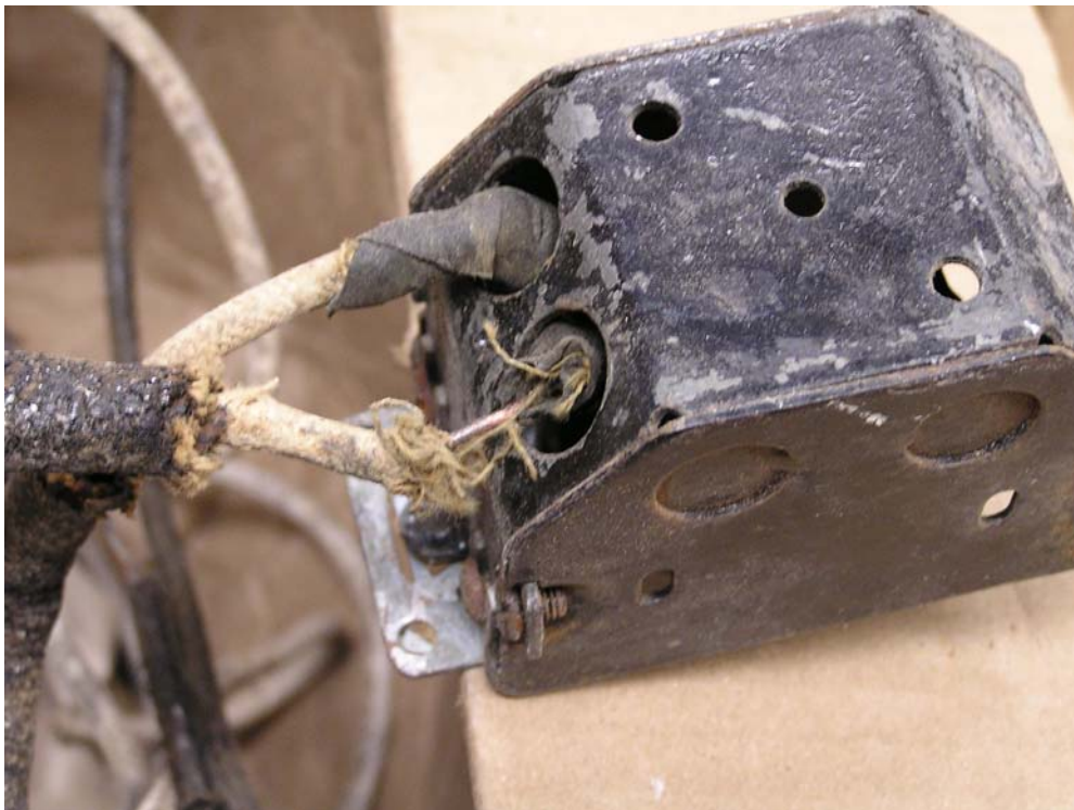
Fig. 8 – Brittle Knob-and-Tube Wire From House TX-2
