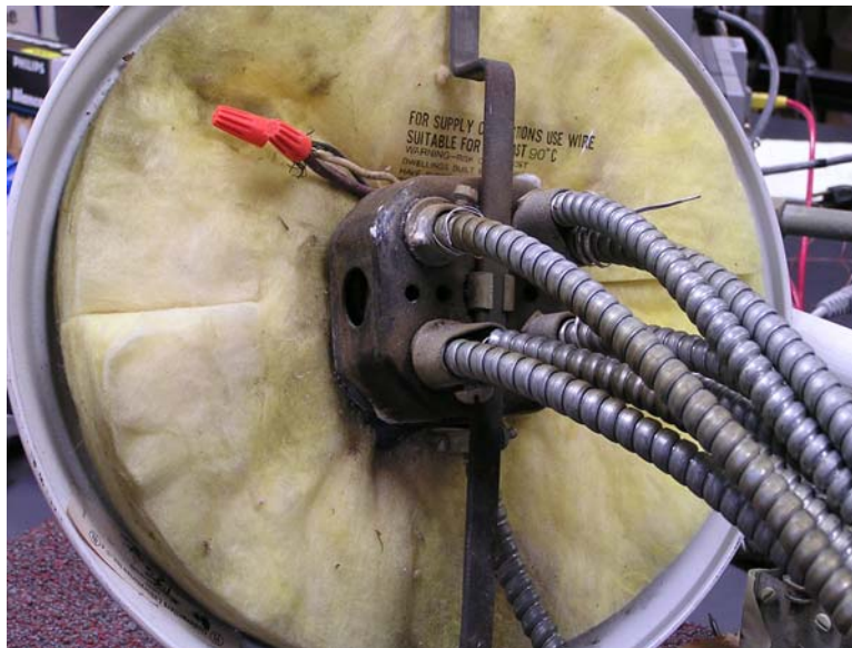
Fig. 26 – From Pilot Project House, 60° C Rubber Supply Conductors
