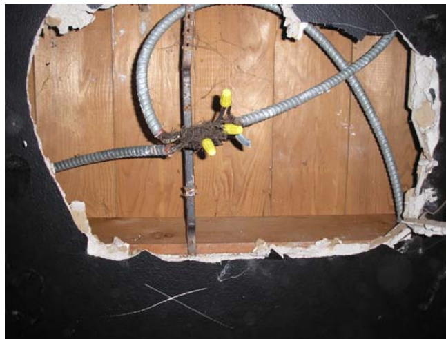
Fig. 35 – House WI-1, Open Splices in Ceiling
