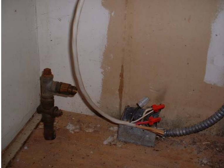
Fig. 34– House AL-1, Unsupported Box (Also No Box Cover)
