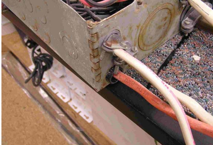
Fig. 36 – House MA-3, Cable Clamp Not Provided
