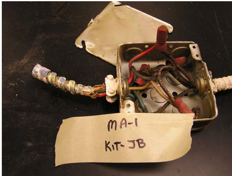
Fig. 38 – House MA-1, No Insulating Bushing Installed With AC Cable
