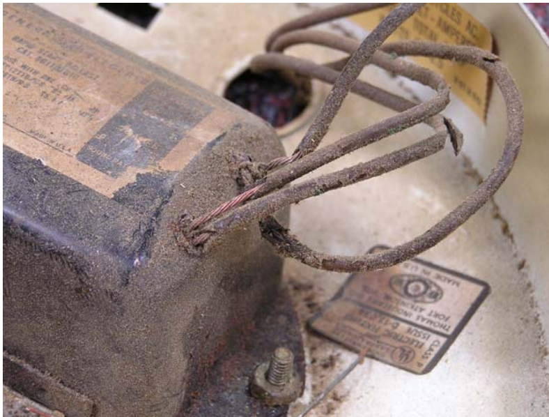
Fig. 21 – House AL-2, Ballast Leads Brittle and Conductor Exposed
