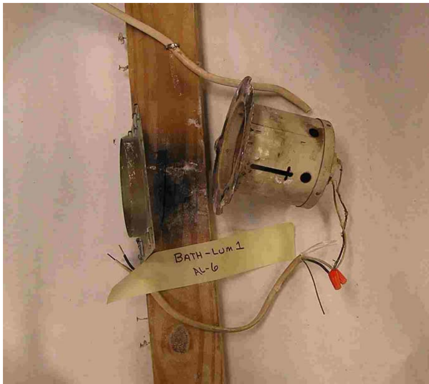
Fig. 22 – Recessed Luminaire From House AL-6
