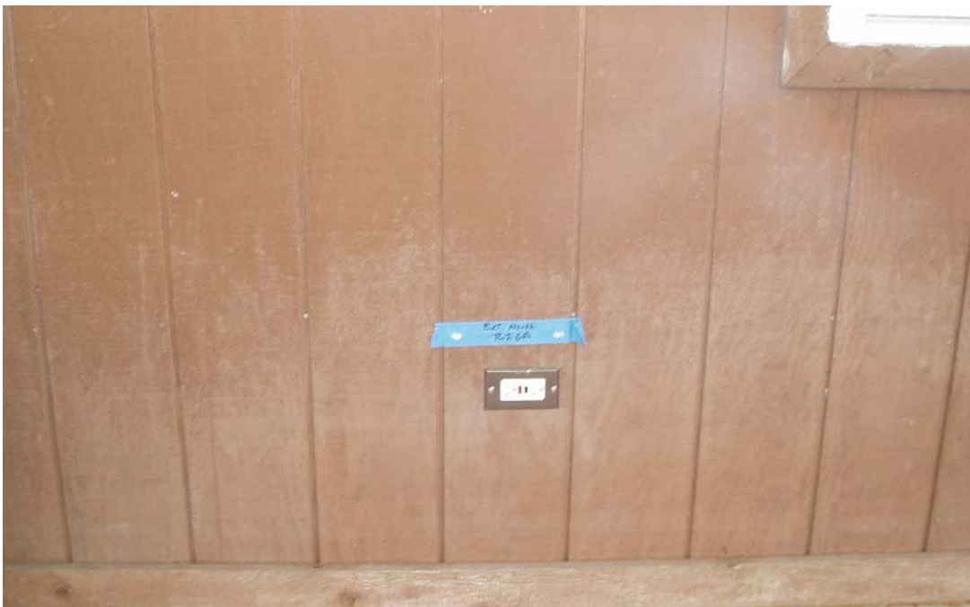
Fig. 25b– House IL-5, Non-Operational GFCI Receptacle With No Outdoor Faceplate or Box Cover (closer view of Fig. 25a)
