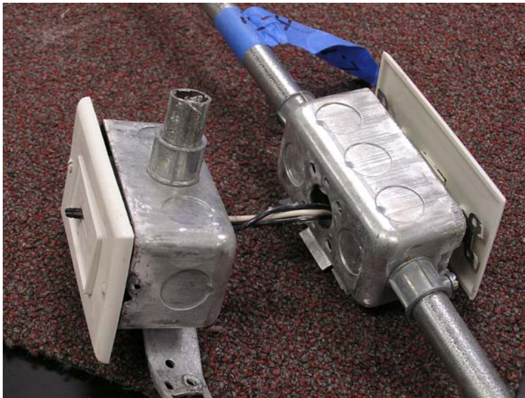
Fig. 33 – House IL-4, Open Conductors In Wall Between Boxes
