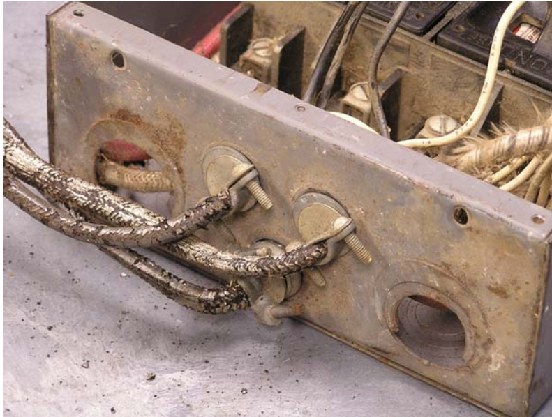
Fig. 27 – House AL-3, Unused Openings in Enclosure
