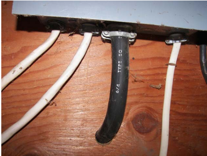
Fig. 40 – House NY-2, Type SO Flexible Cord From Panelboard
