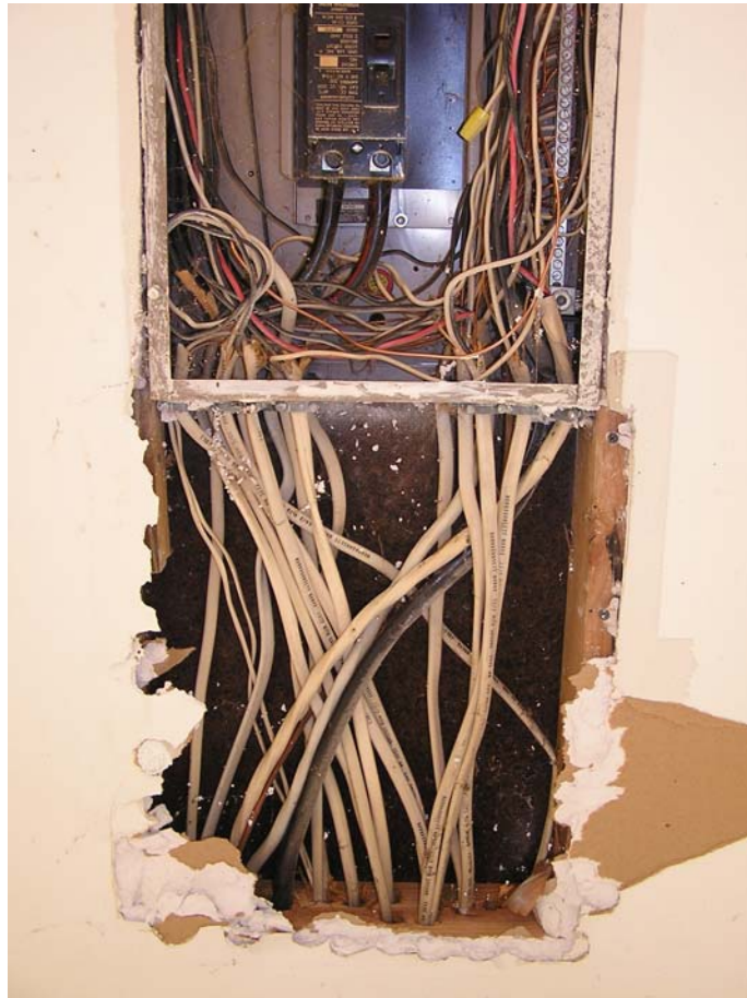
Fig. 6 – NM Cables From House VA-3
