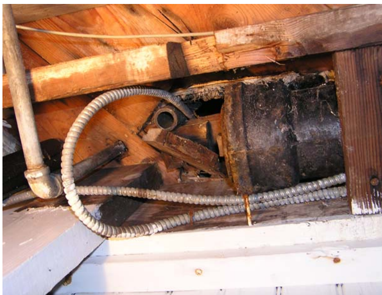
Fig 4 – AC Cable From Basement of House IL-1 With Some Corrosion
