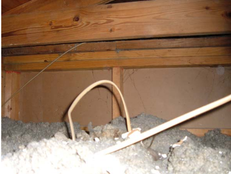
Fig. 43a – House AL-6, Thermal Insulation Above Recessed Luminaire
