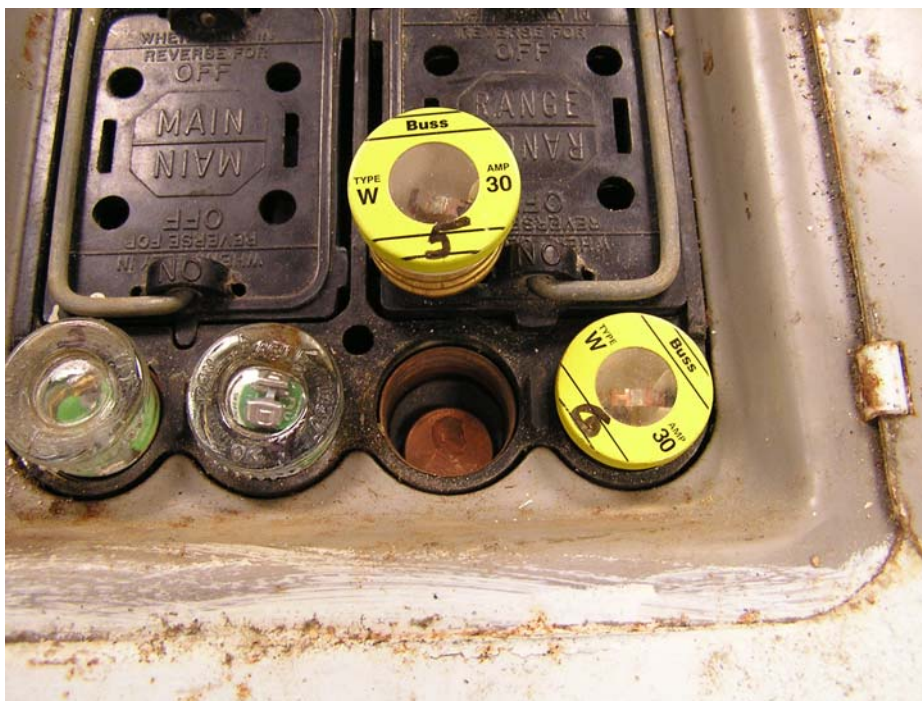
Fig. 13 – Penny Found Behind Blown Fuse at House AL-9
