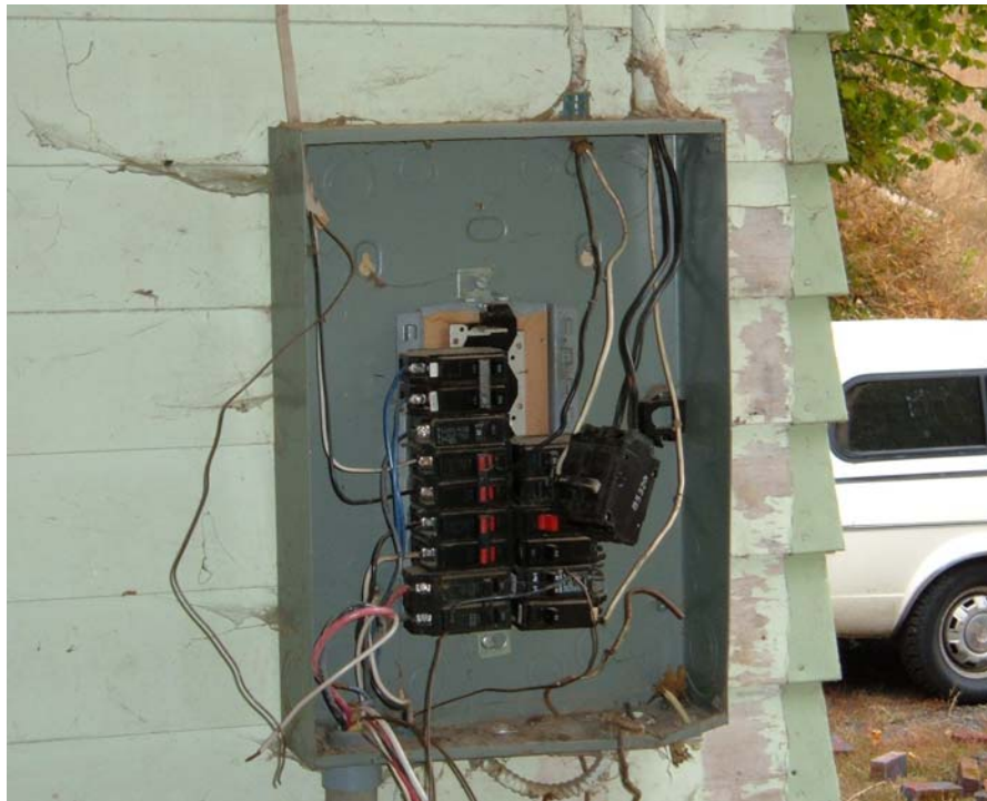
Fig. 30 – House OR-1, Main Disconnect Outdoors
