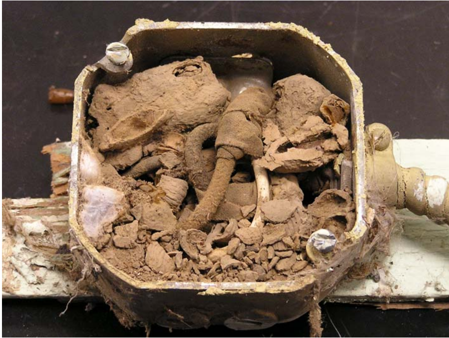
Fig. 23 – Junction Box From House OR-1
