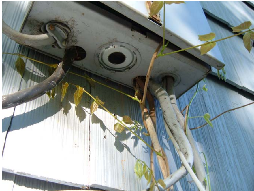
Fig. 14 – Service Enclosure From House AL-8
