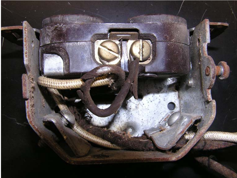
Fig. 7 – Brittle Conductor Rubber Insulation From House AL-7
