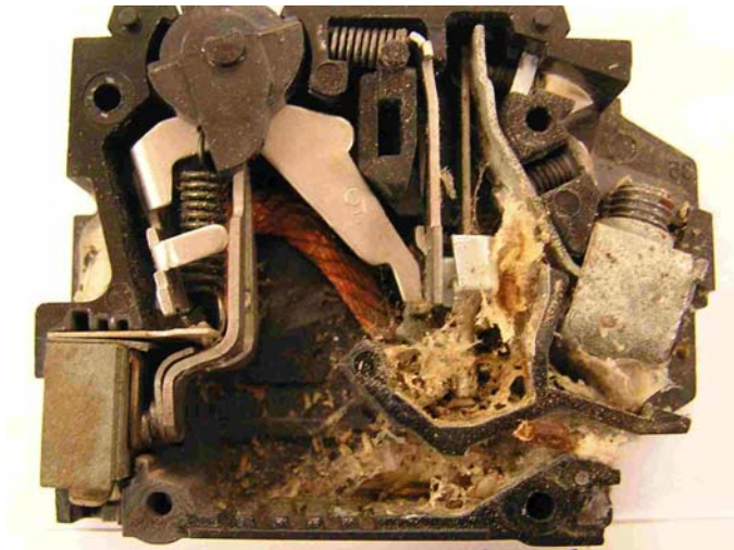
Fig. 16 –House AL-9 Breaker 5-7, Insect Nesting
